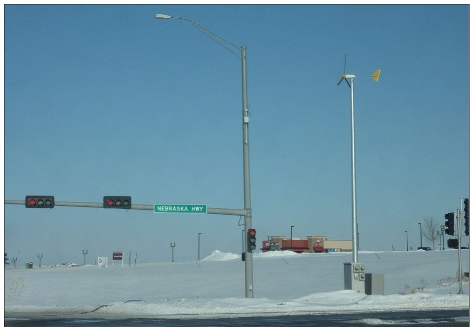
Wind generator and control system at 84th St. and Nebraska Highway 2 in Lincoln, NE. (Photo: Courtesy of Univ. of Nebraska, Electrical Engineering Dept. )
